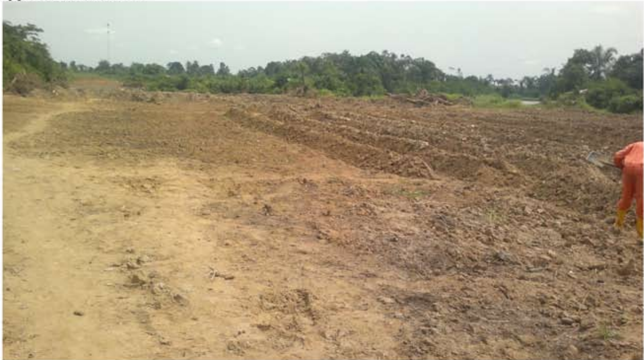
Nigeria Shell spill site final handling of the soil before application of OSE II
